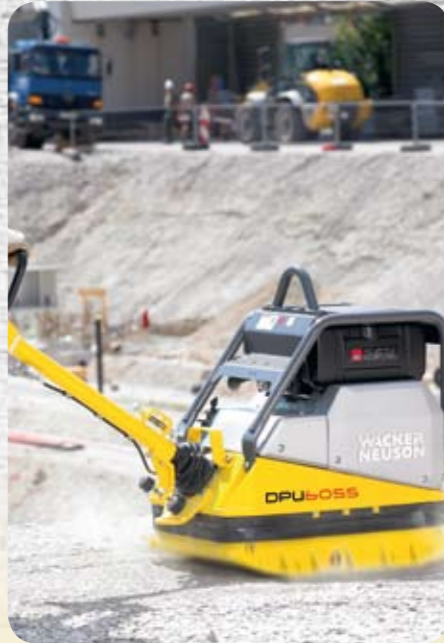
Step 2: The floor is prepared and is compacted before work continues. Depending on the size of the area, Wacker Neuson can offer a wide range of vibratory plates.
