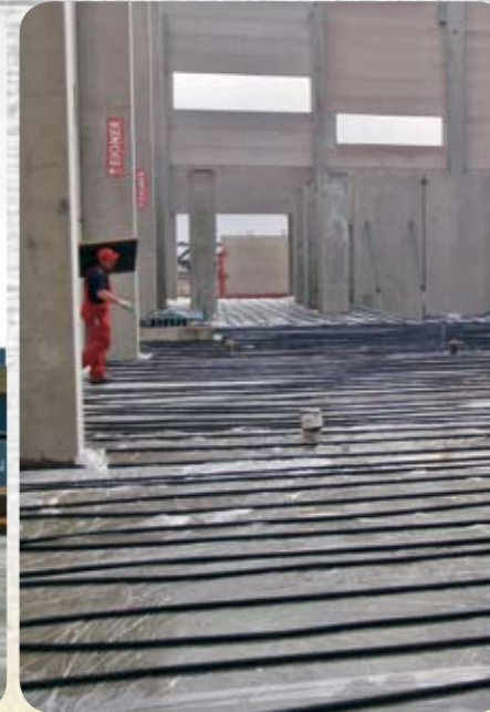
Step 9: Aftertreatment prevents excessively fast cooling and drying of the concrete during the curing process. The Wacker Neuson E 700M surface heater is ideal for this process, as it guarantees a stable setting process thanks to its heating power across a wide area.
