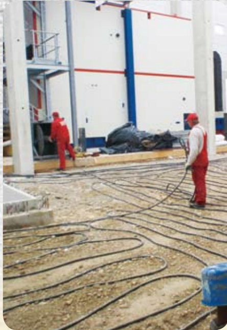
Step 1: Depending on the temperature situation, the floor must have been defrosted and heated prior to finishing. The Wacker Neuson E 700M is the perfect piece of equipment to speed up the process here.
