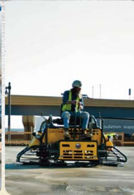
Step 8: Trowels are used to obtain a fine and level surface: first floating, then finishing and finally polishing.
