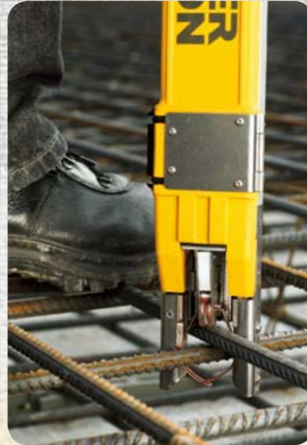
Step 4: The reinforcement is installed and is processed with Wacker Neuson rebar tiers and rebar cutting machines.
