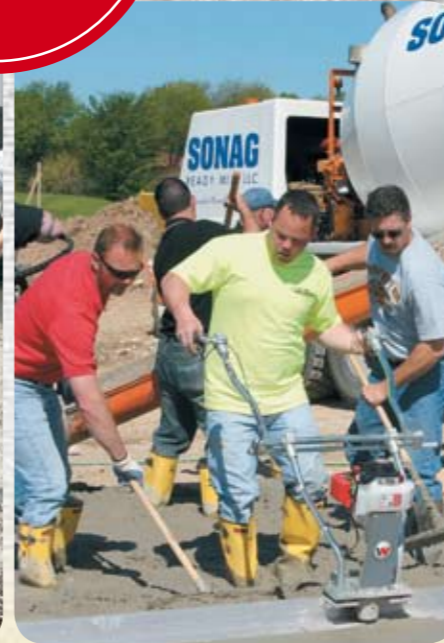
Step 7: The wet screed ensures that the concrete surface is level and that the required height is maintained. The floor is thus optimally prepared for using the trowels.
