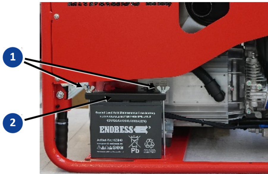
Fig. 9-1 Replacing the starter battery
