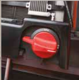
Battery cut-off switch
