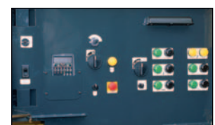
Main Control Panel
