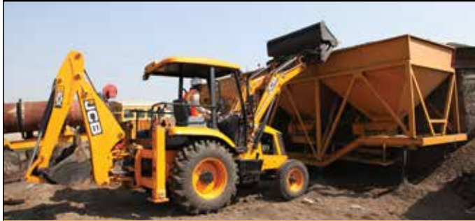
Hopper feeding for ready mix concrete
